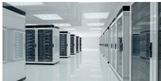
AI Data Servers, Racks, Supercomputing, Infrastructure
