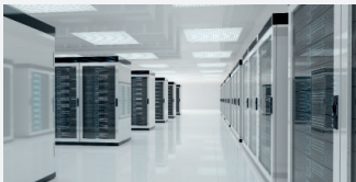
AI Data Servers, Racks, Infrastructure Supercomputing
